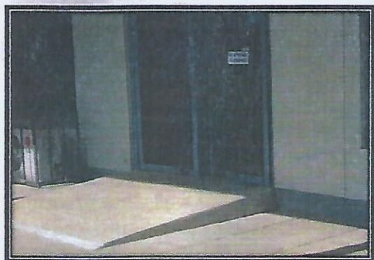
Figure 4: Ramp running directly to threshold of door with no landing
