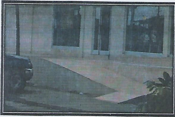
Figure 5: Ramp with no guiding handrails for users Source: Field Survey, 2014.
