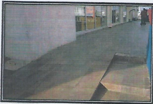
Figure 3: High thresholds at a main entrance doorway Source: Field Survey, 2014.
