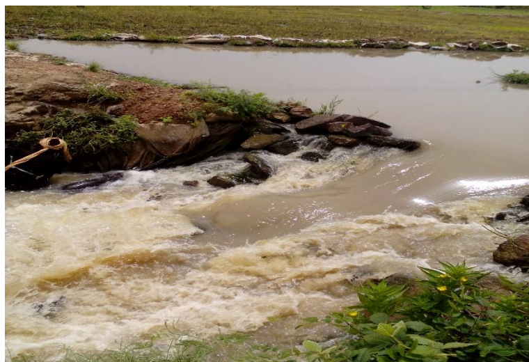
Figure 4: Distribution canal Failure in Kontagora scheme.
