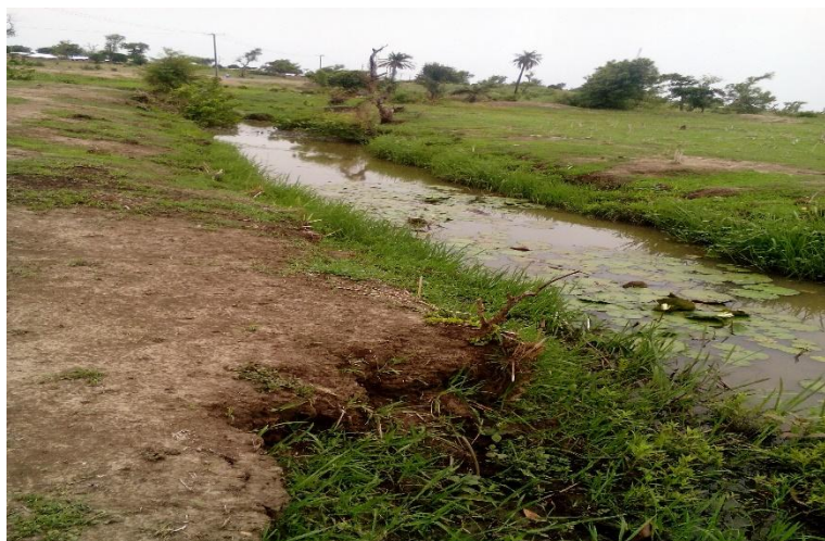
Figure 3: Some section of distribution channel overgrown by weeds.
