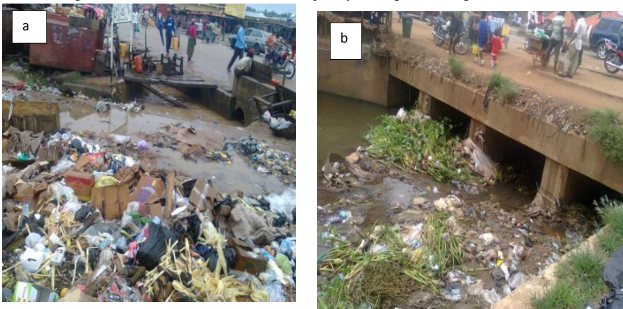
Fig. II a and II b: showing the dumping of solid waste into the drainage system/channels in the study area. (Source, fieldwork)
