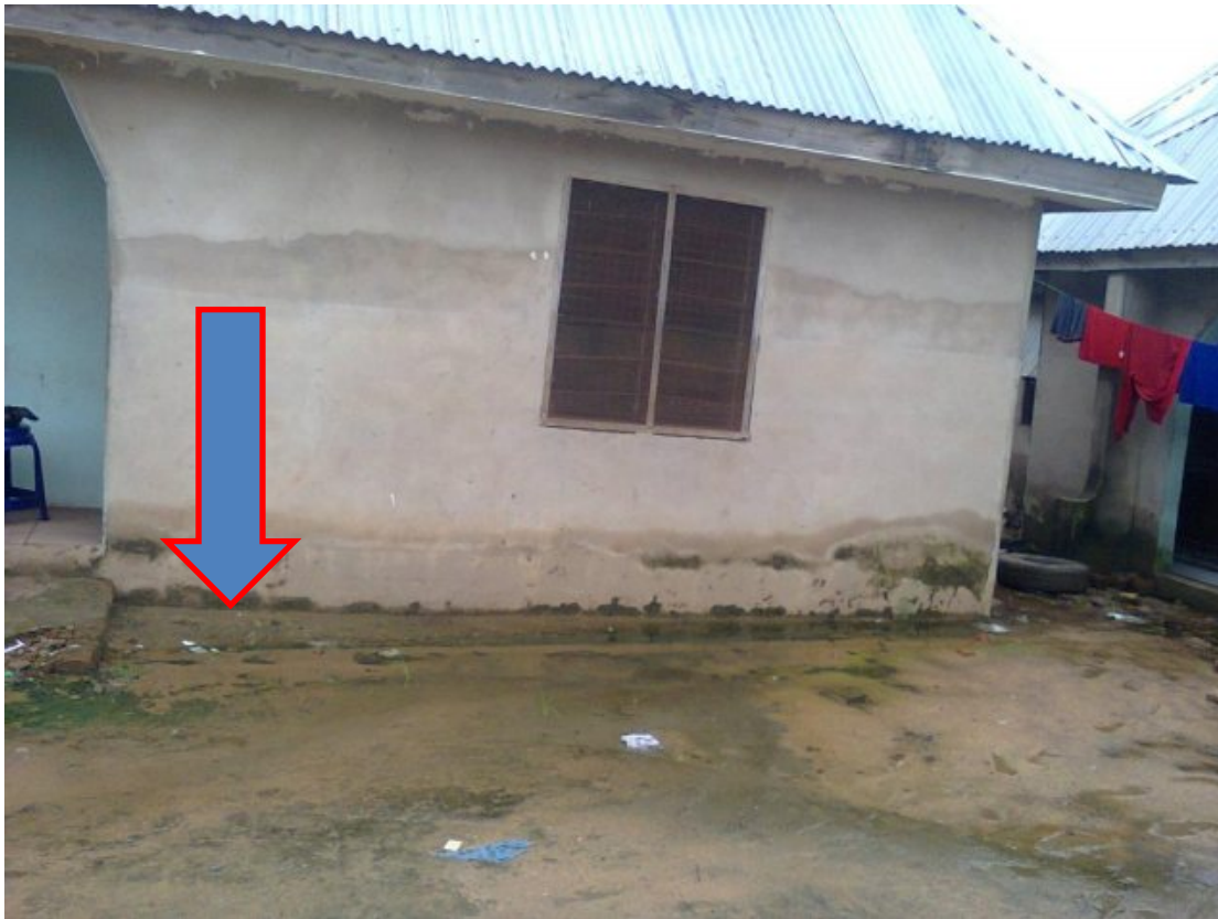
Fig. V: imprint of flood on building’s wall, signifying the level or height of flood waters at the time of impact. (Source fieldwork)
