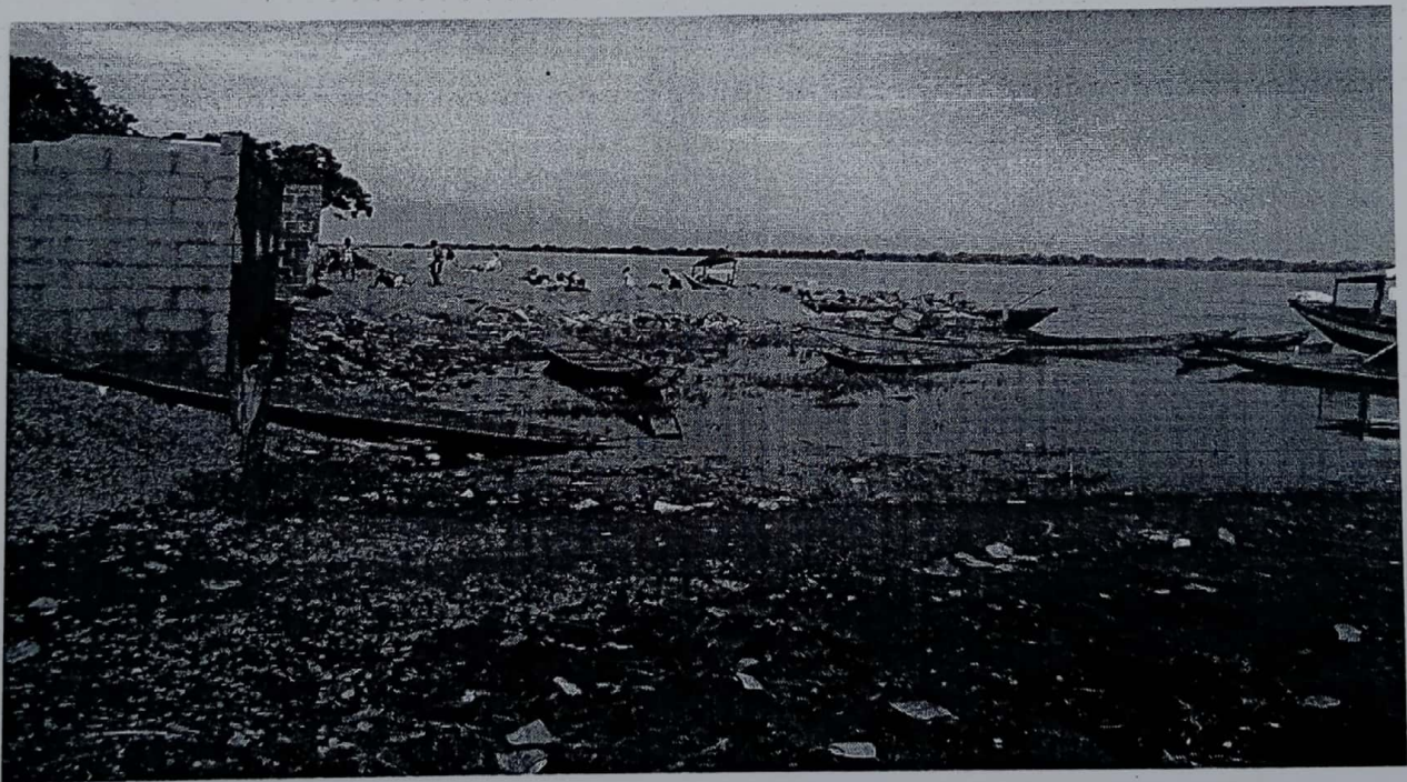
Fig. IV: shows an ongoing construction on the bank of River Benue (source fieldwork)
