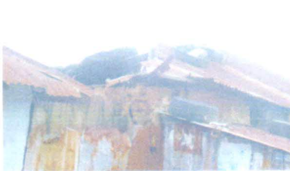
Plate 1c: Rainstorm hazard in Dutsen Kura
