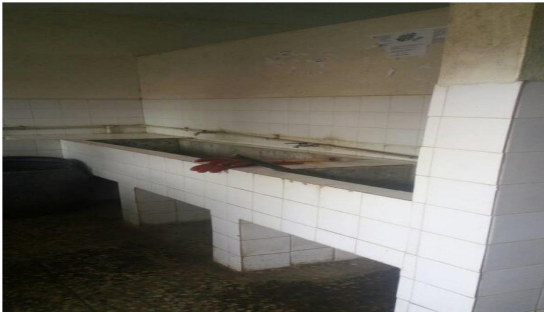
Plate 2 Dilapidated bathrooms in Hostel
