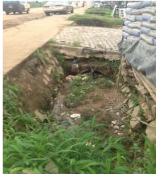
Plate 2: Blocked drainage in public housing Source: Field survey, 2019
