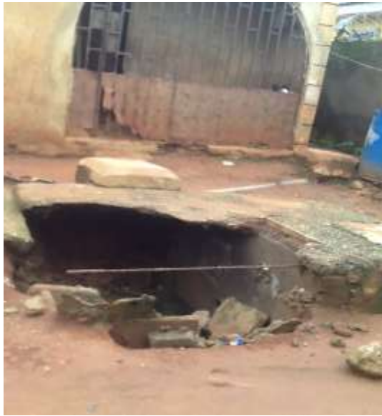
Plate 1: Dilapidated septic tank Source: Field survey, 2019
