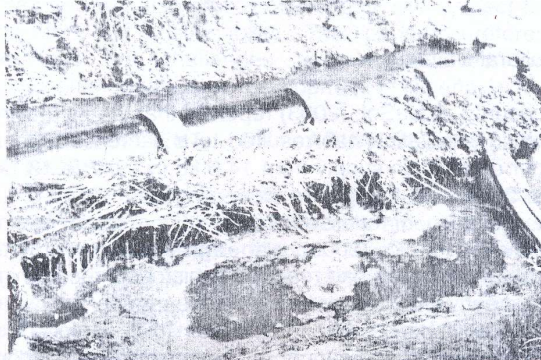
Fig 2 Blocked sewer line
