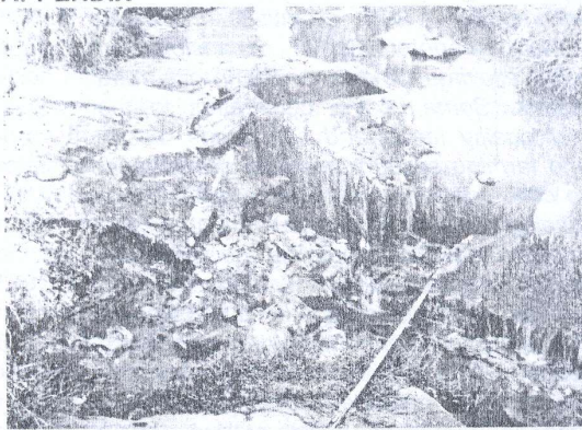
Fig 1 Multiple line Joint man hole
