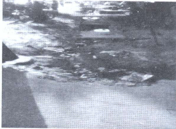
Figure 1: showing filled drainage system along Mypa road due to lack of adequate maintenance of the drainage system and provision of refuse dump sites, culverts constructed for easy passage of traffic and human have collapse further hindering the free flow of water in the drainage system vehicles and human. An example of this is that found along Ibrahim Sarki Randan Ruwa in Bosso.
