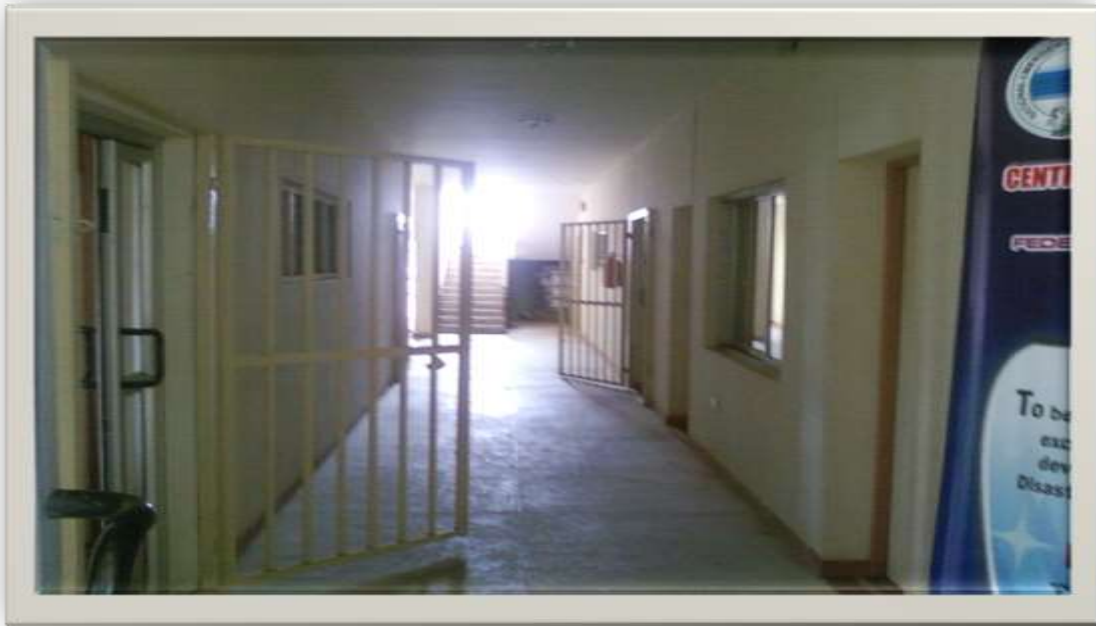
Plate VII: Showing the Corridor with Inadequate Lighting and Ventilation
