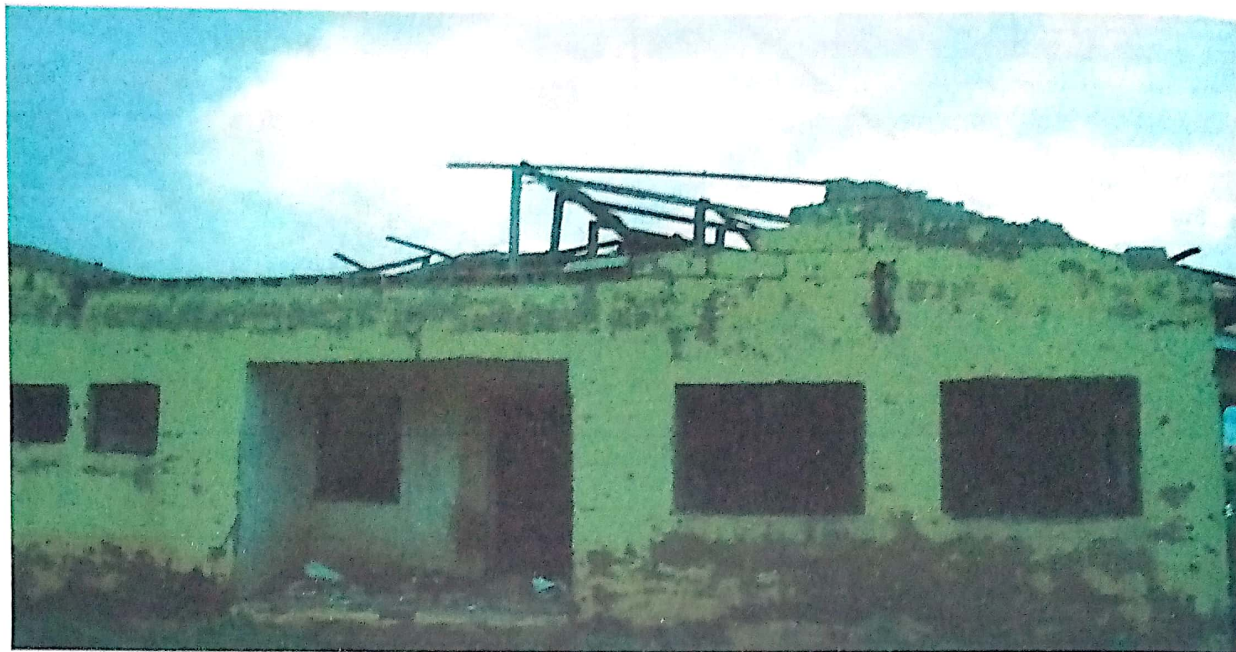
Plate 1: Poorly constructed unit
