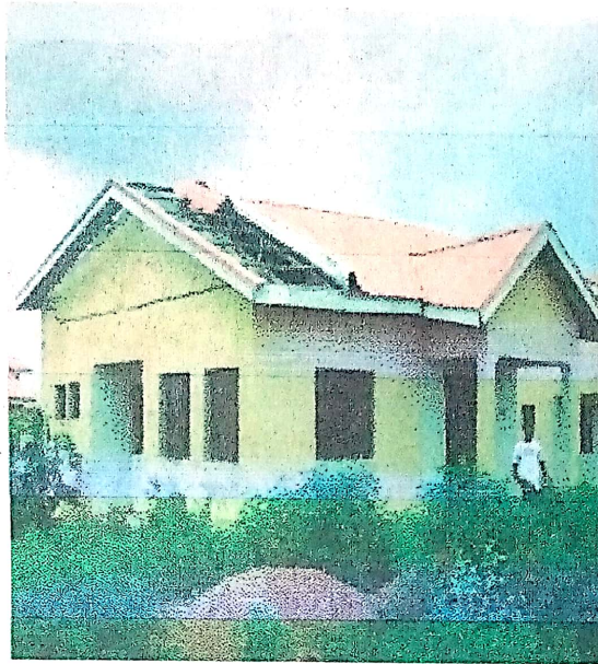
Plate 3: Cracked wall Source: Authors field work, 2010
