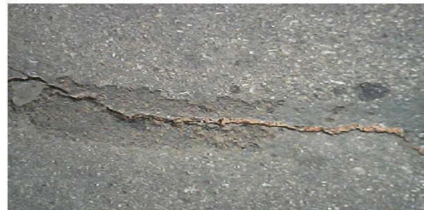
PLATE II: HORIZONTAL CRACK ON A PAVEMENT CONSTRUCTED ON BLACK COTTON SOIL
