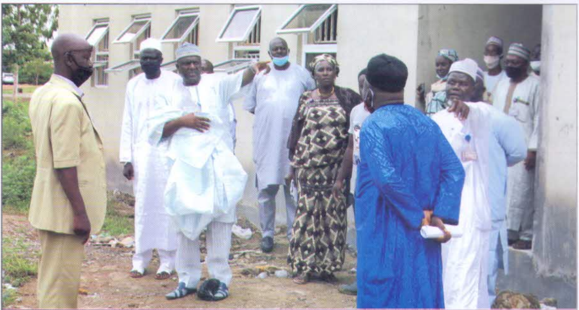
The VC, Prof. Bala (m) explaining a point to the contractor at the site while others watched with keen interest.
