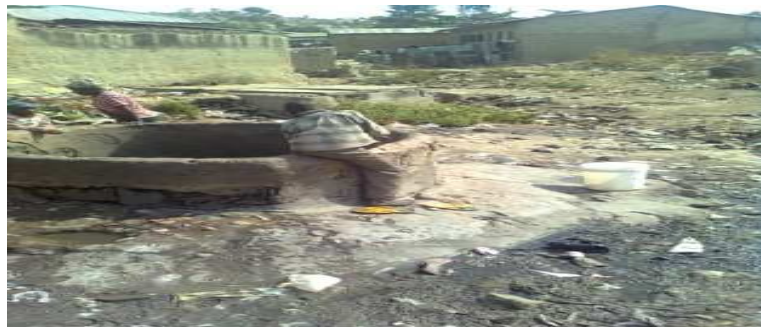
Plate iv: Drainage system close to an open well in Angwanbiri
