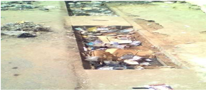
Plate i: Showing filled Drainage system along Mypa road
