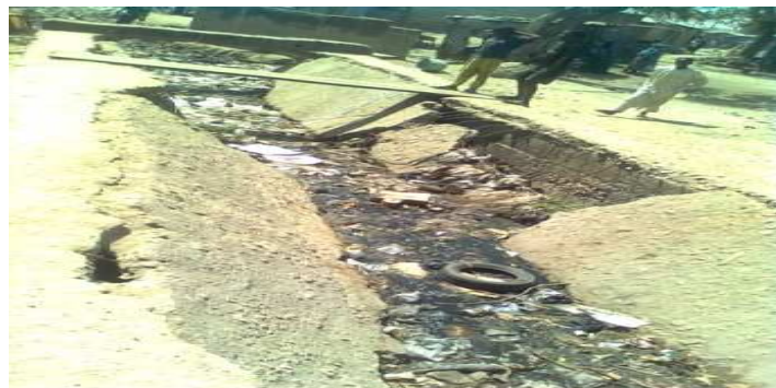
Plate ii: Showing a collapse Drainage system at back of Emir’s house
