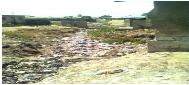
Plate iii: Broken down fence wall along one of the drainage channels
