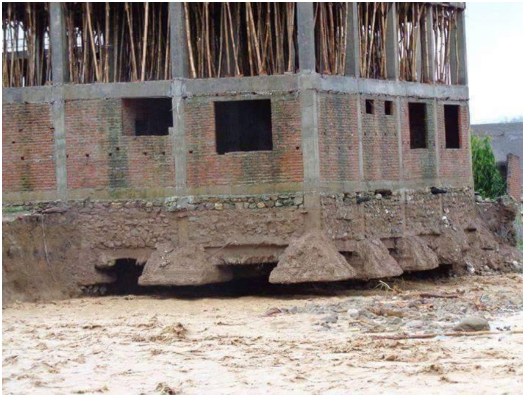
Plate I: Eroded Foundation of an uncompleted Building due to Flood
