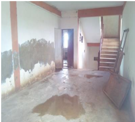
Plate 3: emergency stairs way of Male Hostel F.U.T Minna Gidan Kwano Campus Source: field work (2015)
