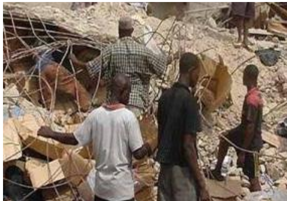
Plate 1.: A collapse building due to use of sub-standard material. Source: Amadi, Eze, Igwe, Okunlola & Okoye(2012 )
