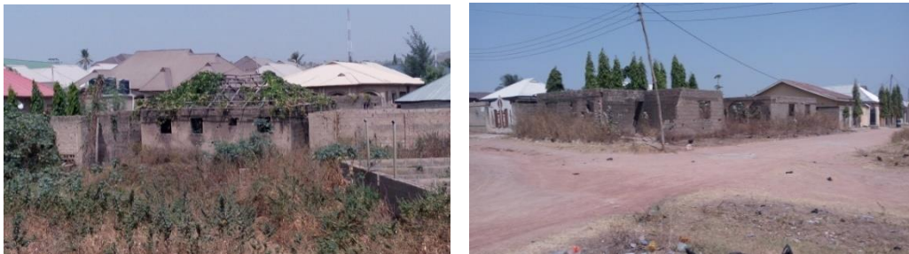
Plate 1 and 2: abandoned residential buildings in F-layout extension and London Street respectively where residents in neighbouring buildings have complained about the series of attacks by snakes and scorpions and foul odour.
