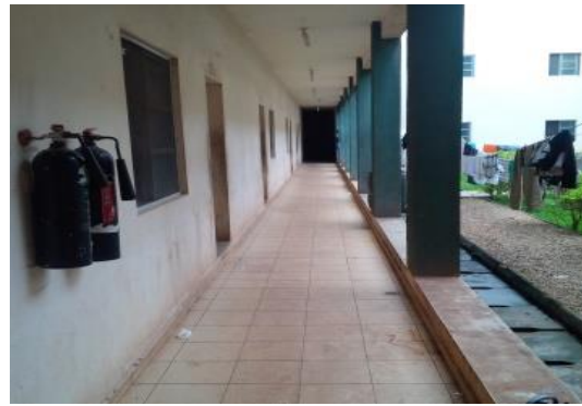
Plate 6: Fire Safety Equipment At Corridor Of Male Hostel Ibrahim Badamasi Babangida University. Source: Field Work (2015)
