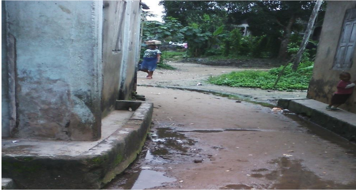
Raised slabs constructed round the building using a concrete mix of shells, gravels and cement to guard the foundation in Apkaekpehem Community
