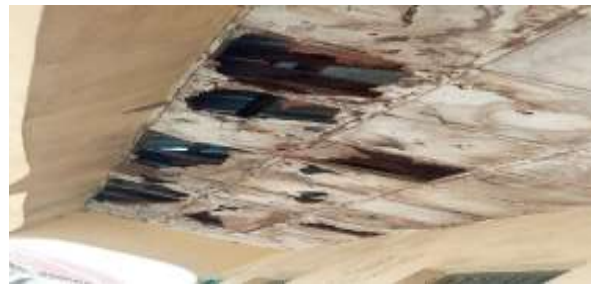
Plate 6: Showing decayed ceiling
