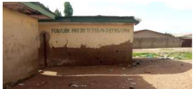
Plate 8: Showing washed out walls
