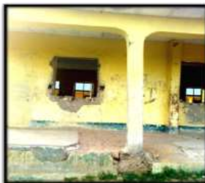
Plate 16: Dilapidated windows and
