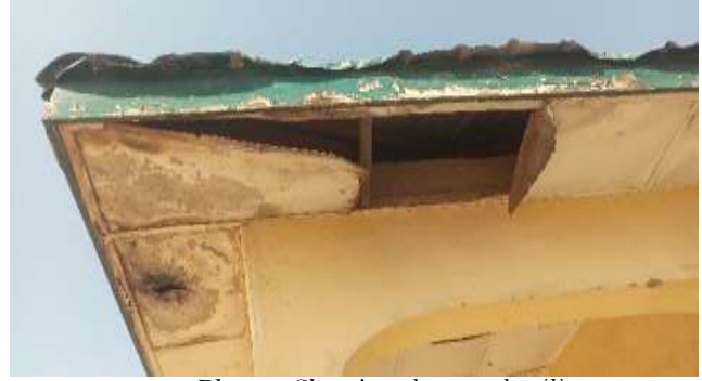
Plate 4: Showing damaged ceilings
