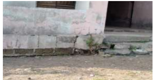
Plate 15: Showing broken riser
