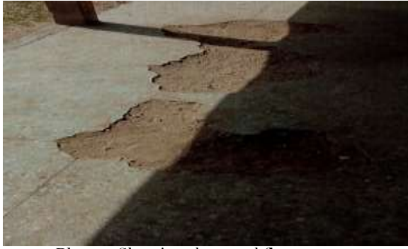
Plate 3: Showing damaged floor
