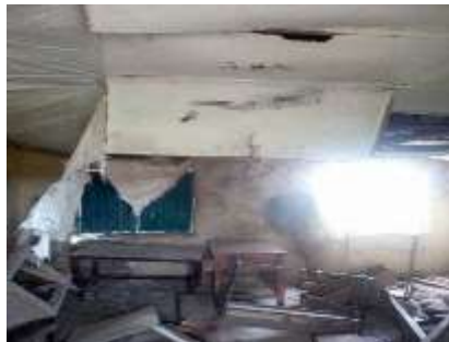
Plate 11: Showing dilapidated Classroom
