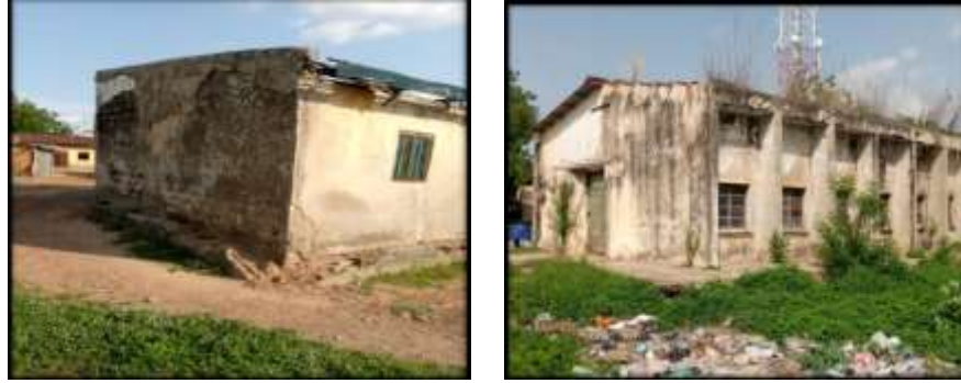
Plate 18: Dilapidated view of the building at Tunga
