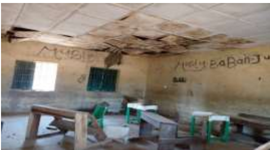
Plate 7: Showing decayed ceiling
