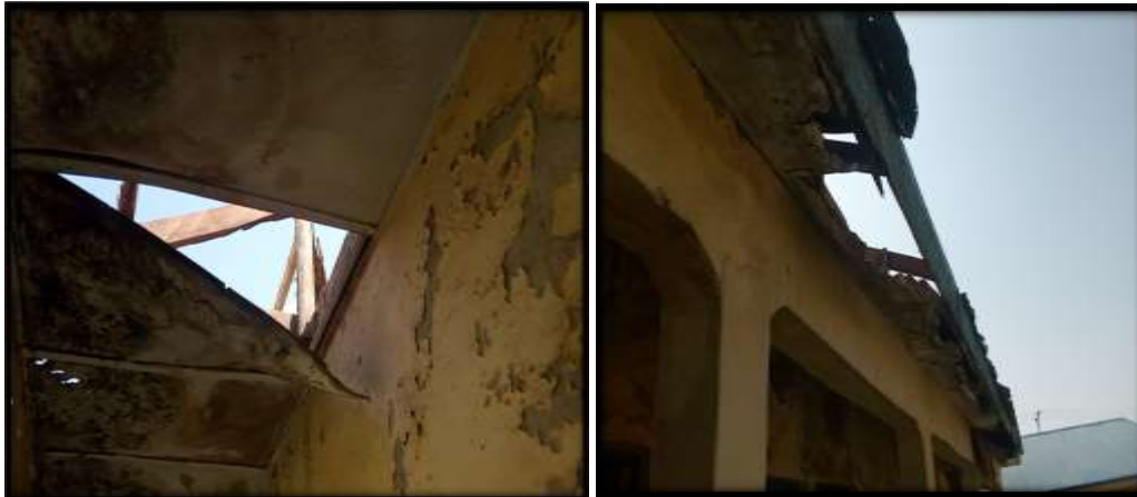
Plate 19: Completely damaged ceiling and roof.at Gidankwano L. E. A Primary school
