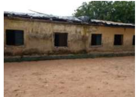
Plate 10: Damaged Roof and Structure
