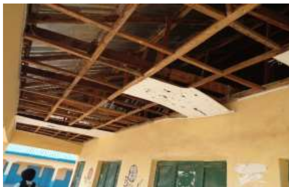
Plate 1: Showing damaged ceilings
