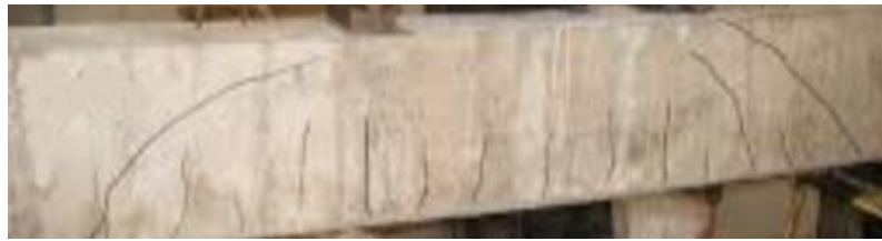
Fig.2(a). Experimental Cracking Pattern in Control Beam
