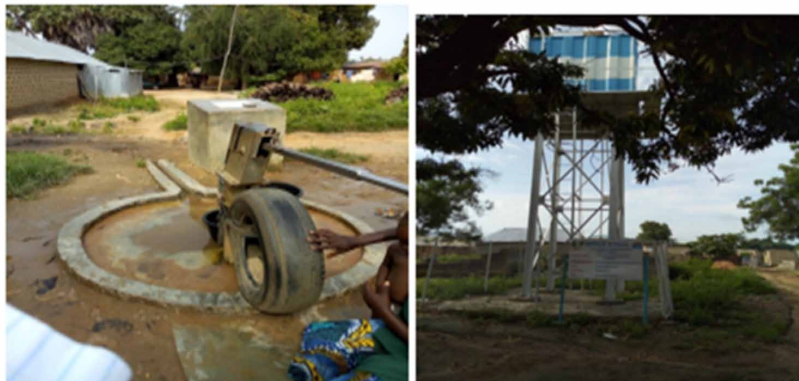
Figure 8. Water infrastructure condition Gidanmangoro and Garatu, respectively
