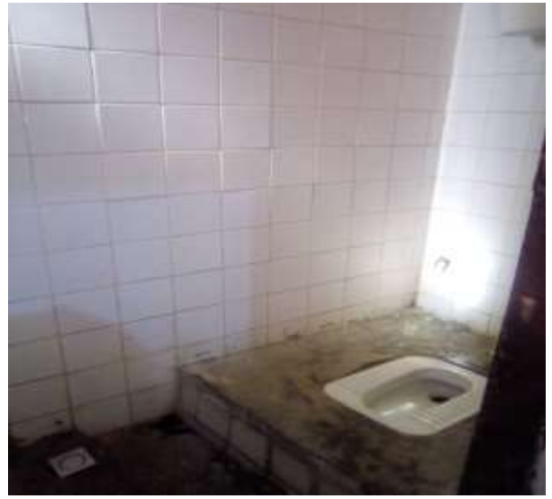
Figure 4.7 Gidan kwano Female Hostel Toilet
