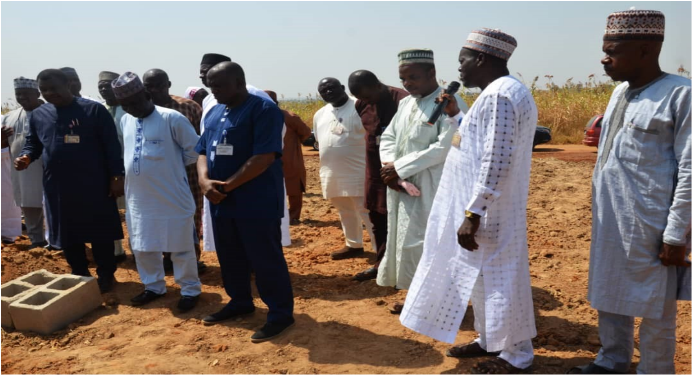
The Chairman of the cooperative Dr Abubakar Usman, speaking at the project site shortly before the foundation laying.
