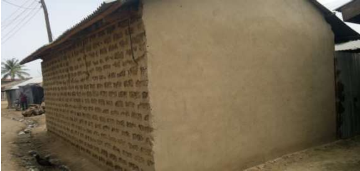
A Typical House built with straw bricks in Matumbe area of Minna, Niger State, Nigeria
