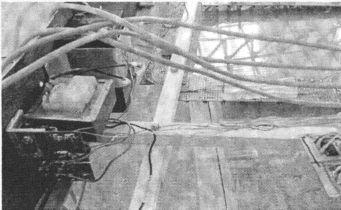
Power section, with back-up battery close to a.c transformer, and heat sink for regulator ICs.
