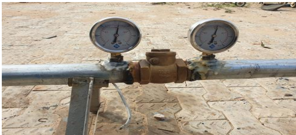
Plate III: Pressure gauges on the experimental test rig
