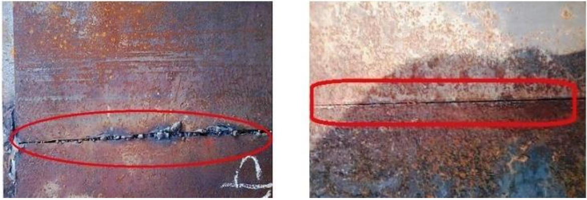
Figure 2.7: Inadequate Joint Penetration Source: (Anand, 2017)
