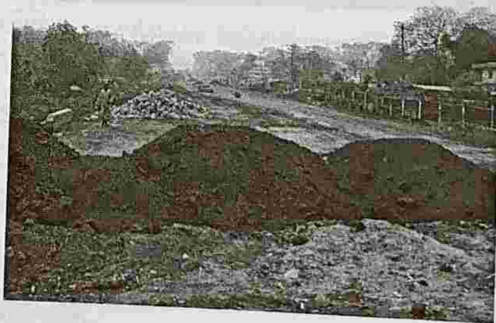
Plate 3. Showing road blockage without any signage. Source:- field work (April 2009)
