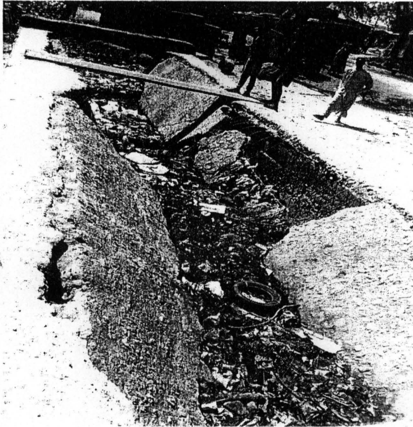
Plate 4.2. Showing a collapse Drainage system at back of Emir's house
