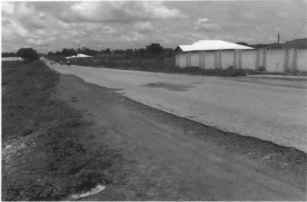
Plate V The Washing away of Road Surface due to Erosion
