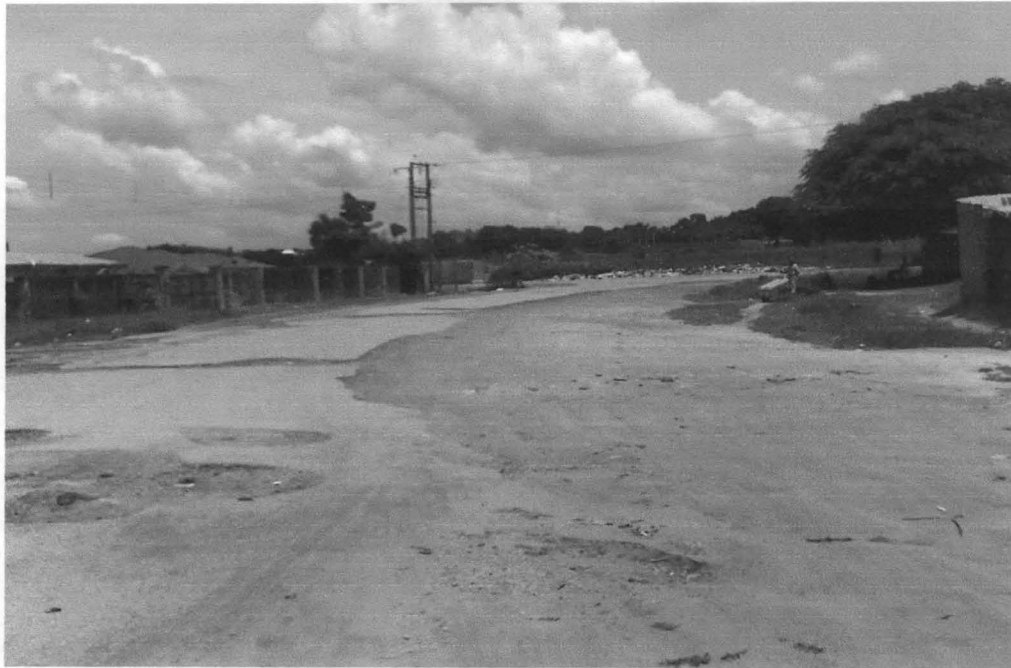
Plate IX An Estate Road Washed away by Erosion ,Bosso Estate .
