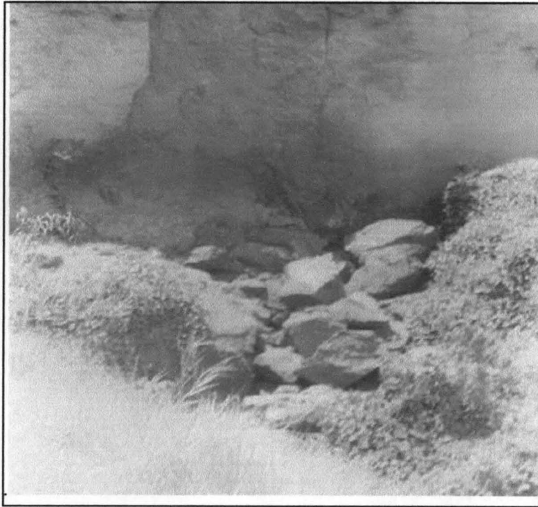
Plate 4.2: Expansion of sidewall
