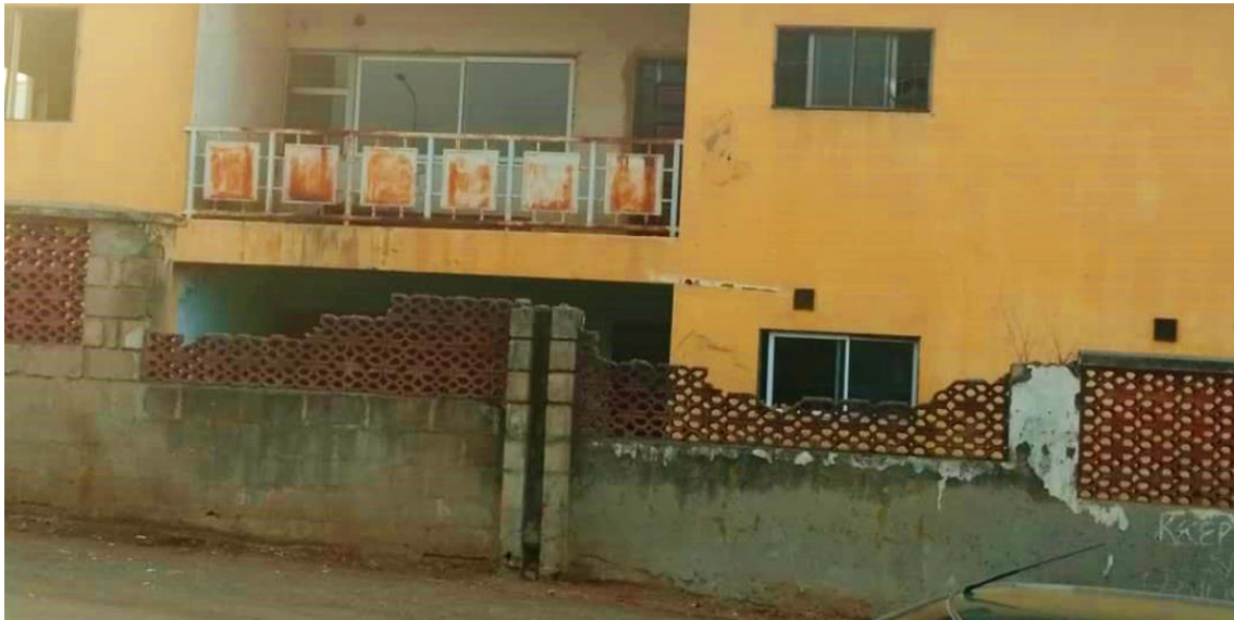
Plate I: Image of Building Affected by Obsolescence in Garki Abuja.
