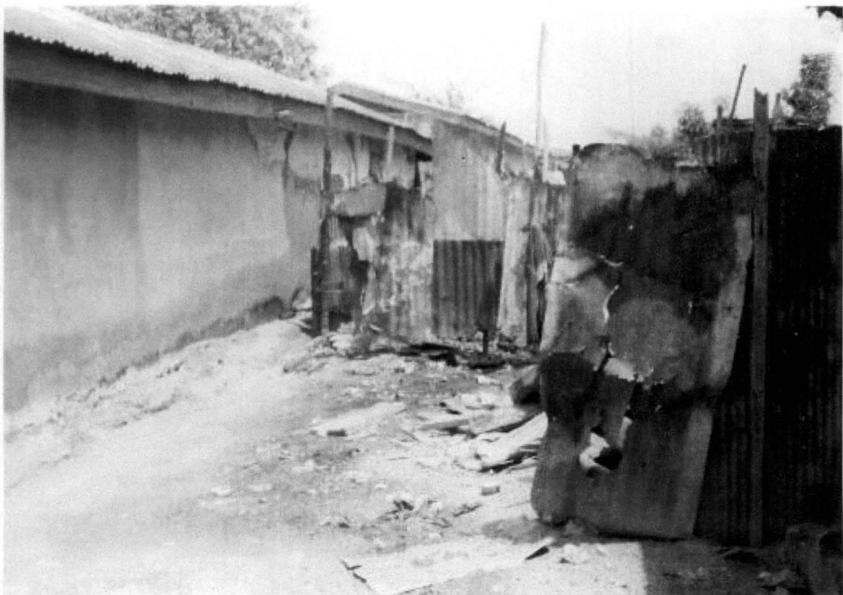
Plate VIII: Showing a typical bathroom/ toilet provision for buildings in the area
