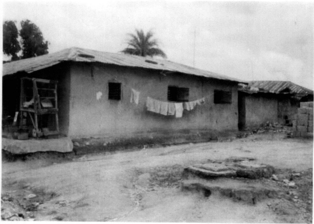
Plate I: Showing inadequate ventilation in a building studied
