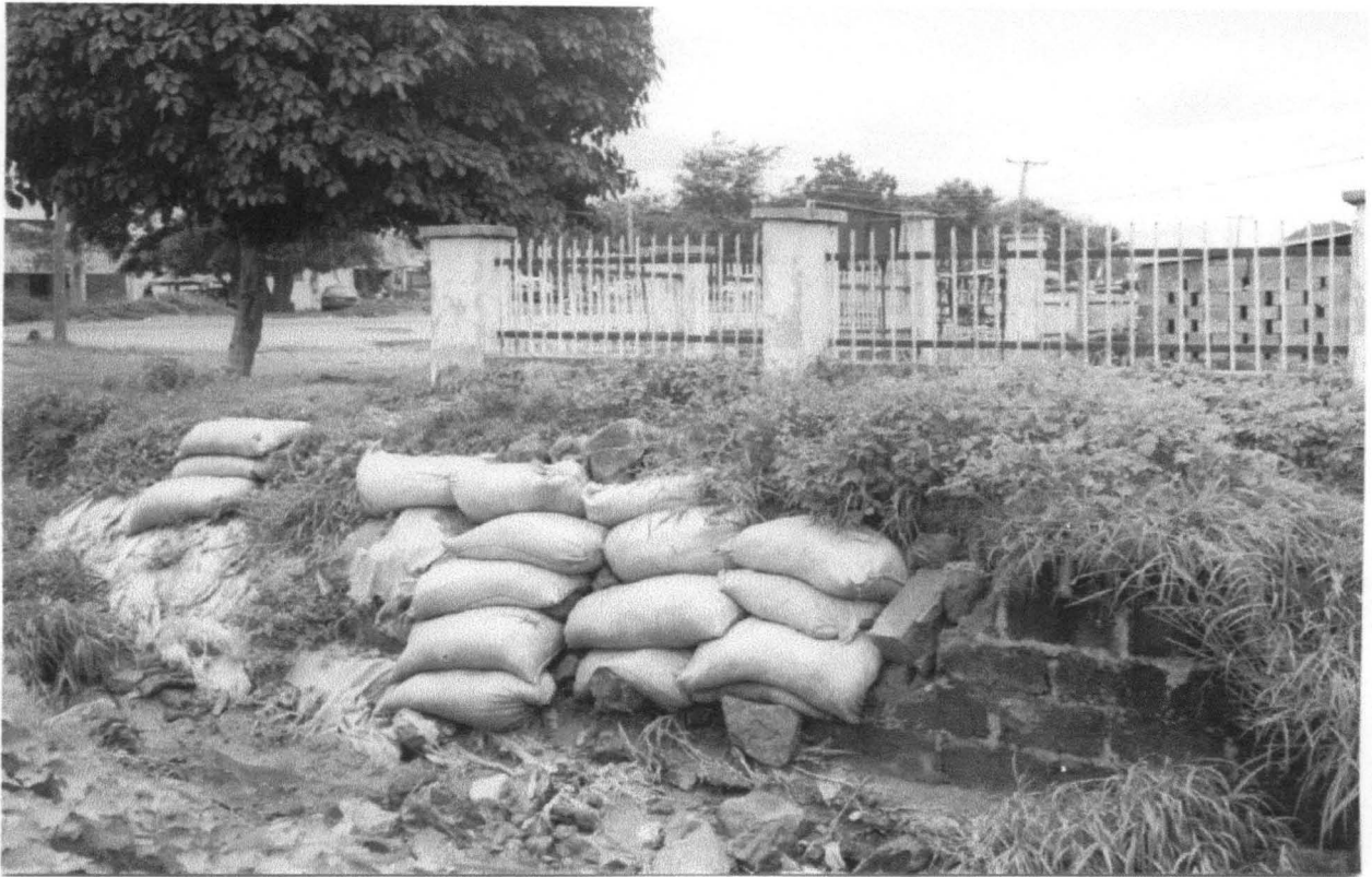
PLATE 5.15: Shows Sand bags were used to present erosion activities
