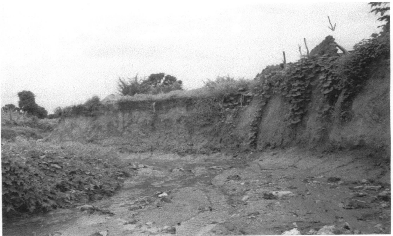
PLATE 5.5 and 5.6: Reveal a part of a house fence and a loom collapsed due to eroded portion of the land surrounding the house at Kwangwara study area SOURCE: Field Survey, 2001
