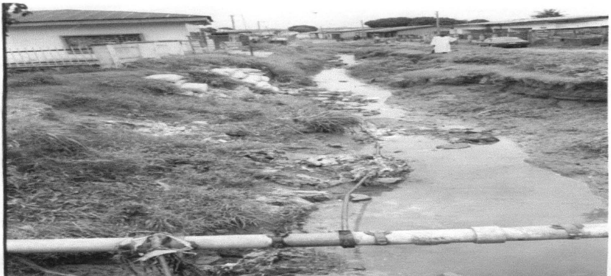
PLATE 5.9 to 5.11: Shows water pipes reveal to the surface due to erosional problem, at water works study area SOURCE: Field Survey, 2001
