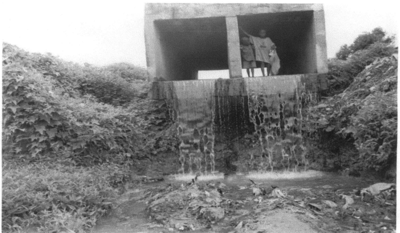
PLATE 5.2: Shows a bridge rendered useless at Unguwar Yamma due to erosion activities SOURCE: Field Survey, 2001
