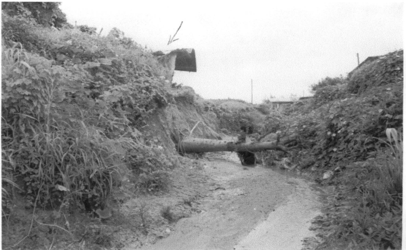
PLATE 5.4: Another house being chopped off by erosion at Unguwar Yamma in Kontagora central SOURCE: Field Survey, 2001
