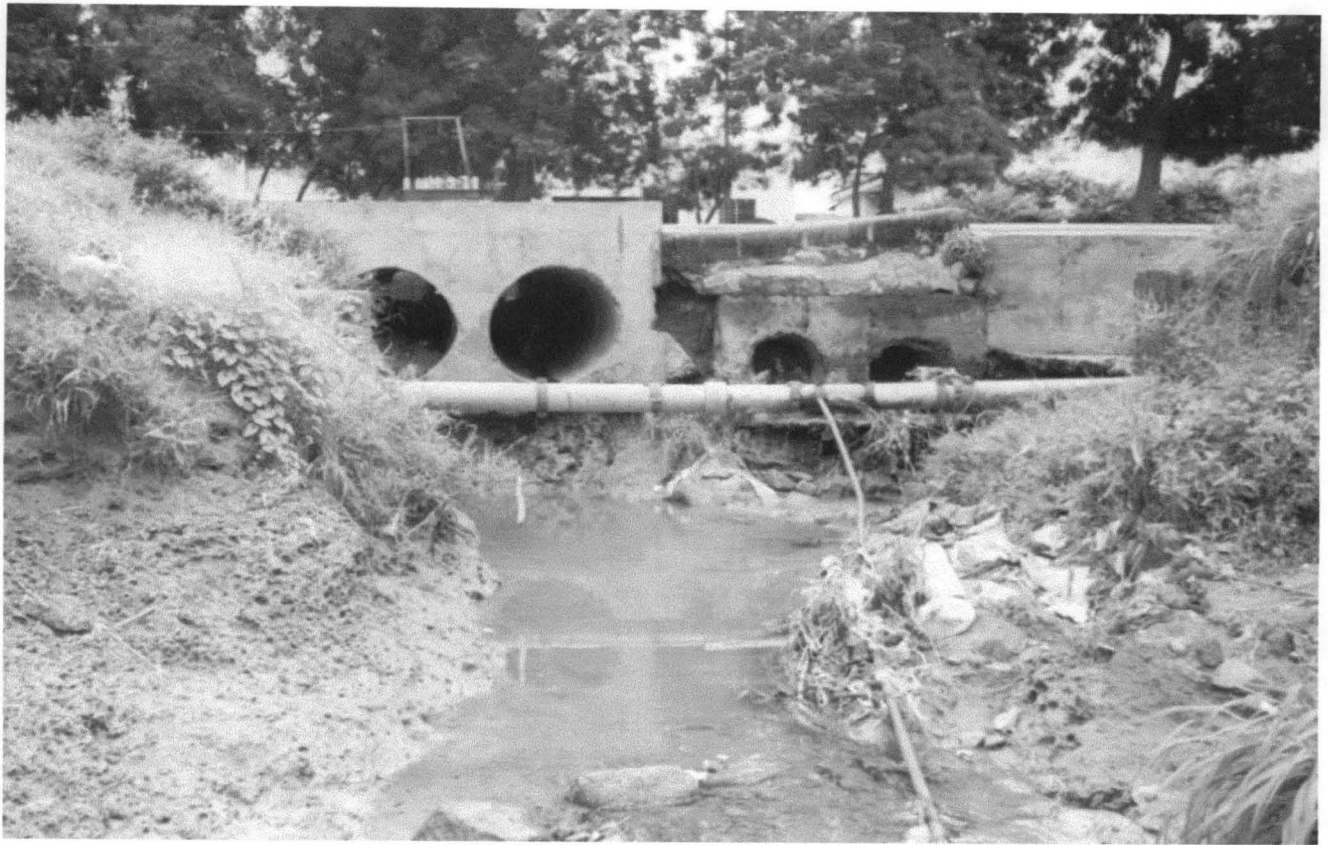
PLATE 5.3: Shows a buried pipe now exposed to the surface as a result of erosion SOURCE: Field Survey, 2001
