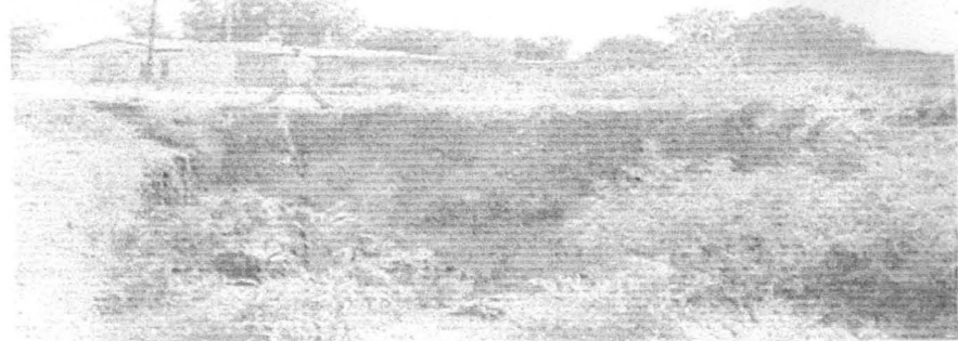
4.2.4: This is as a result of the above poor construction of drainage which led to making this area susceptible to erosion and the menace of land degradation. This is the consequences of lack of E.I.A. (I.s environment impact assessment).
