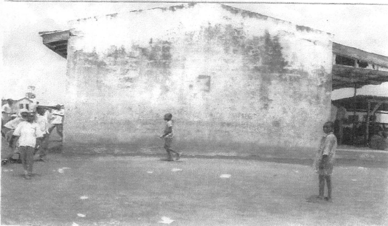
Plate 12: Shows the wall of a Primary School in Chanchaga with washed off paint surface, flaked rendered wall and damped fascia board with decayed ceiling board.
