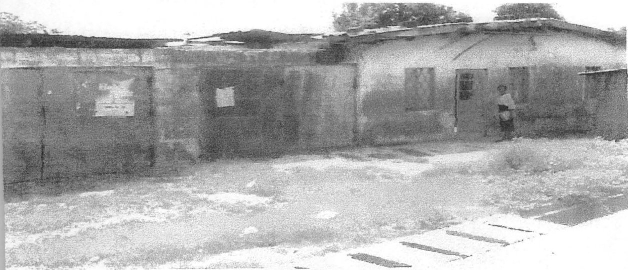
Plate 1: The effect of rainstorm on a house; Wind has blown off Part of the roof, discoloured paint surface, corroded metal gate, roofing timber, fascia, board and ceiling board decayed due to moisture.
