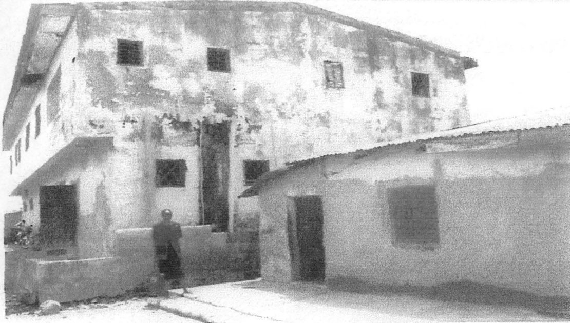
Plate 9: Shows the effect of rain on a storey building washing of the paint and damp penetration at the top part of wall surface.
