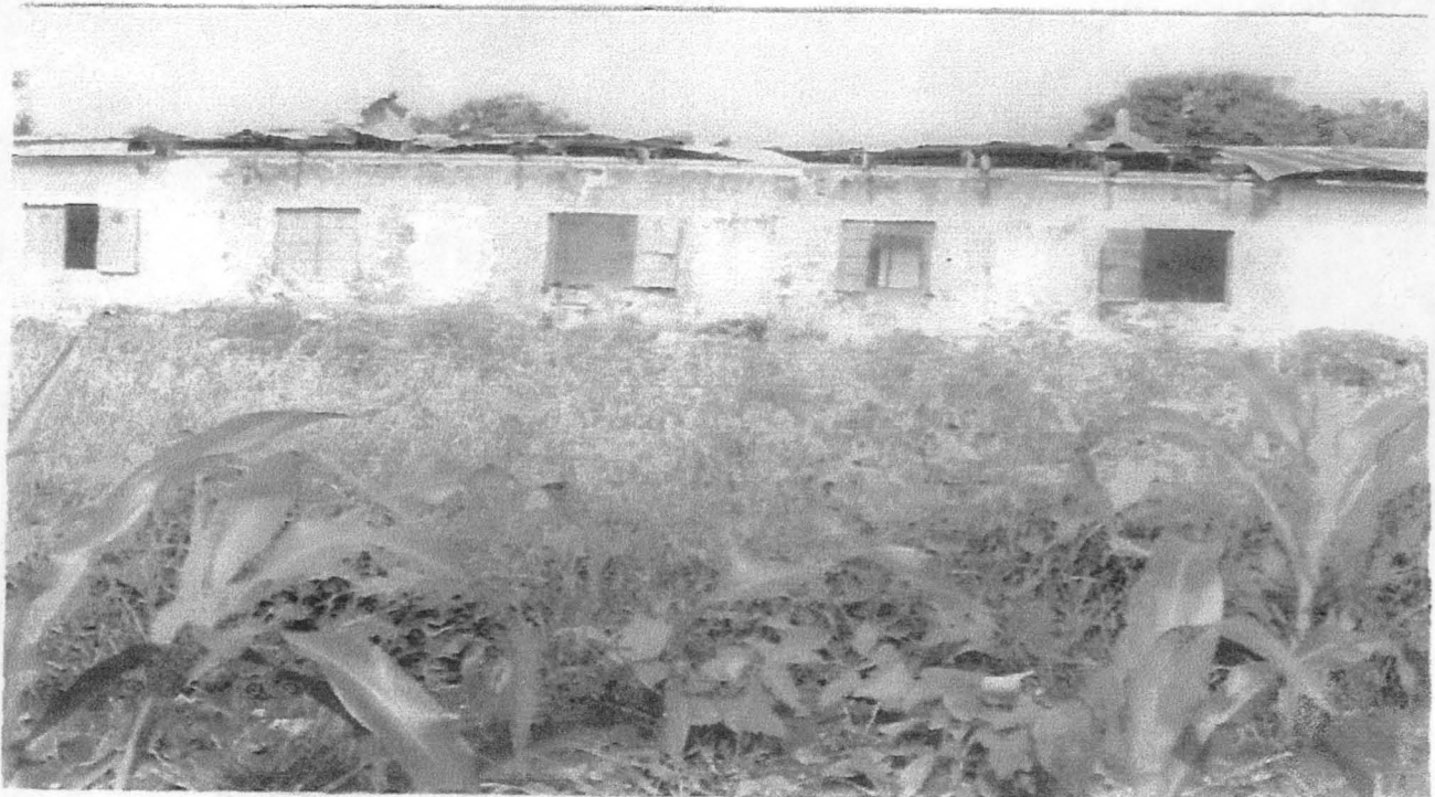
Plate 6: The effect of rain washing away the paint on wall and Wind blowing off part of the roofing sheet. Also part of Fascia board and ceiling board completely falling off in G.T.C. Minna.
