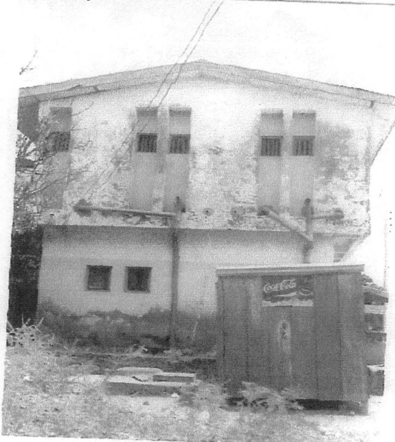
Plate 10: Shows a storey building affected by rainstorm causing discolouration of the wall at the first floor of the building and underground moisture at the ground floor in Chanchaga town.
