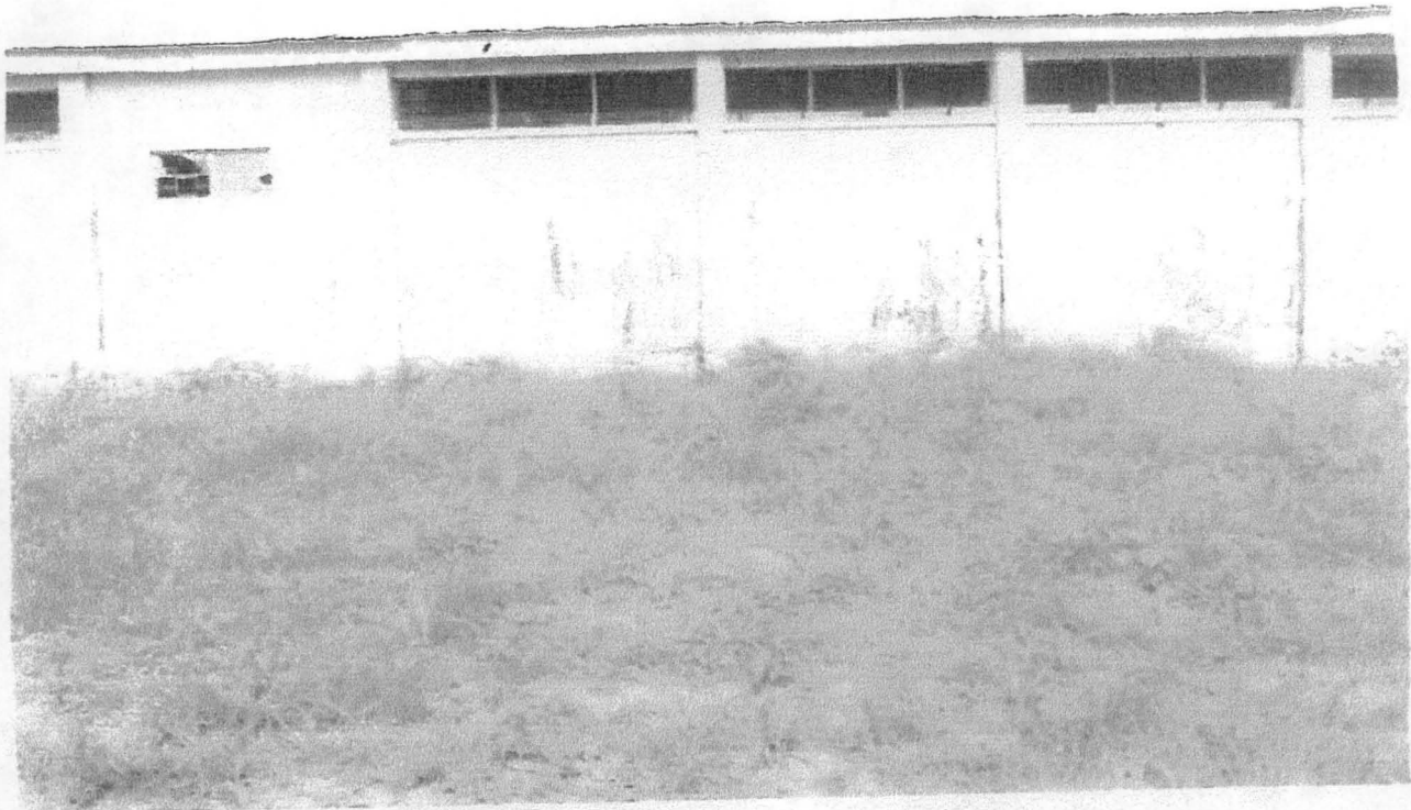
Plate 11: Shows the effect of rain on wall surface washing off the paint on a workshop block in G.T.C. Minna in Chanchaga town.
