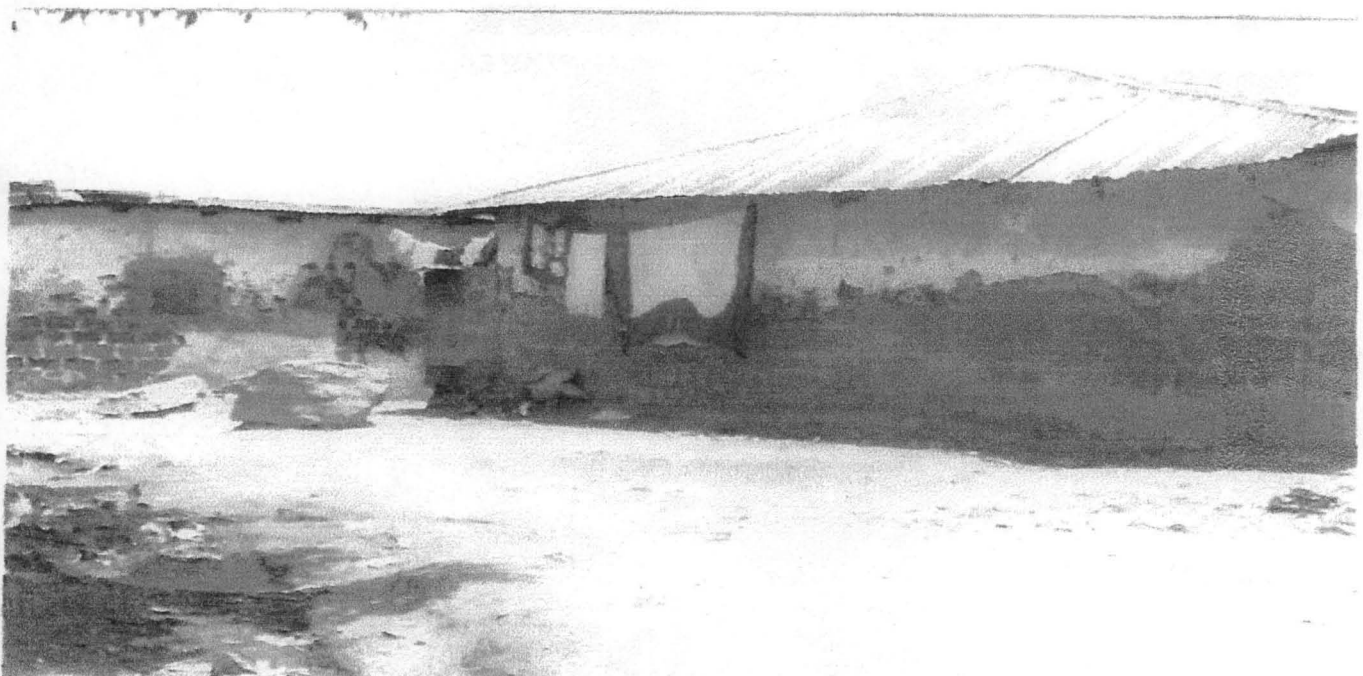
Plate 4: Shows the effect of rain which have wash off the paint and peel of the rendering exposing the mud and sandcrete block in Chanchaga town.
