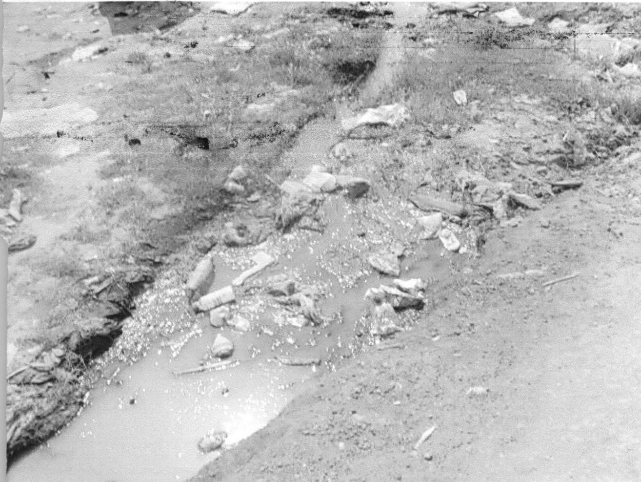
PLATE II: POOR DRAINAGE SYSTEM (SITE A)
