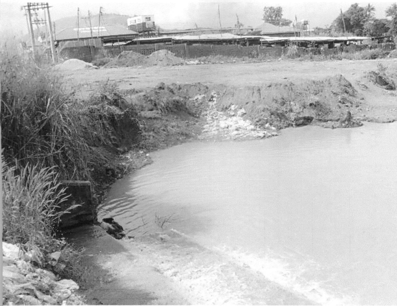
PLATE I: RIVER, DUTSE-JAM, SHOWING BANK EROSION
