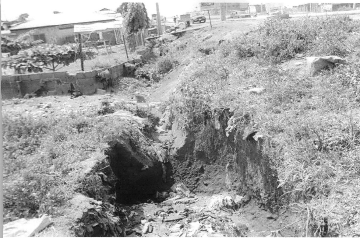
PLATE IX: TYPICAL GULLY EROSION SPOT
