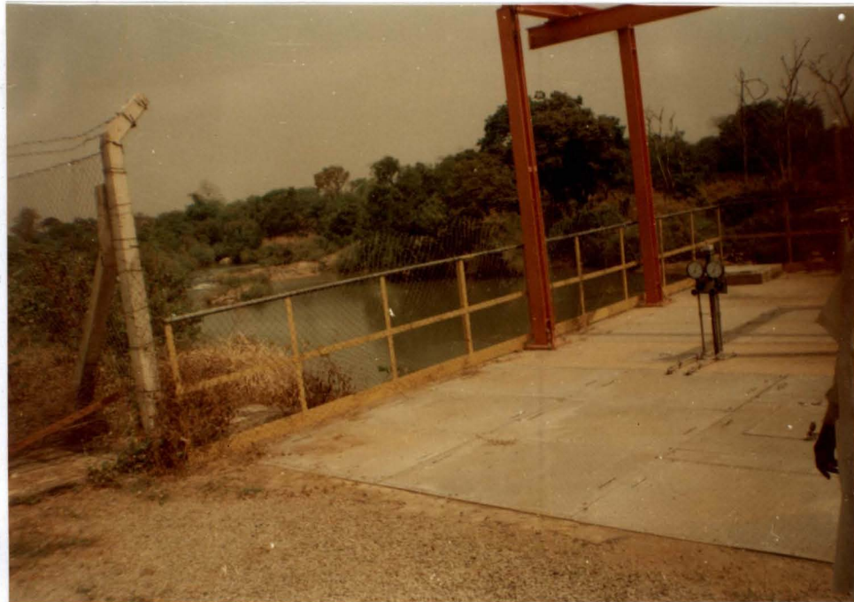
WATER WORKS MAIN SOURCE AND RAW WATER PUMPS MANTLED TO IT.
