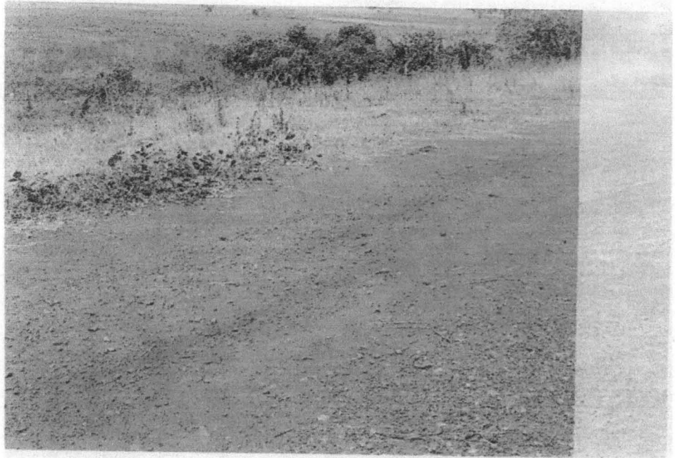
PLATE A:- Dam Embankment with longitudinal crack at chainage 1.6km.
