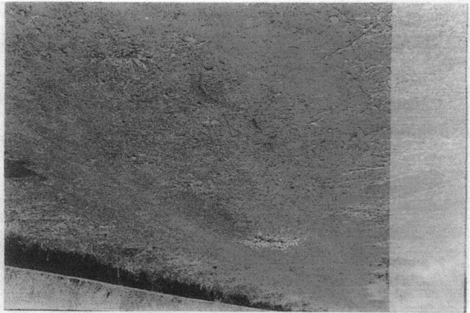
PLATE B:- Dam Embankment with longitudinal crack at chainage 2.5km.
