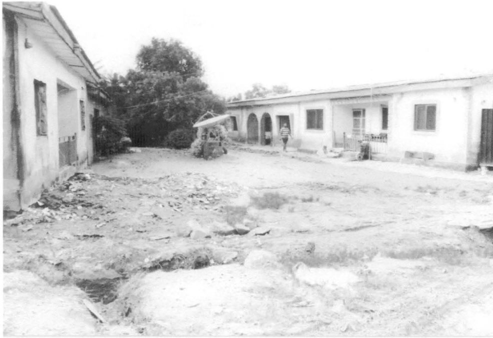
Plate VII: Deplorable state of some of the buildings in F.H.A. estate phase III Kubwa
