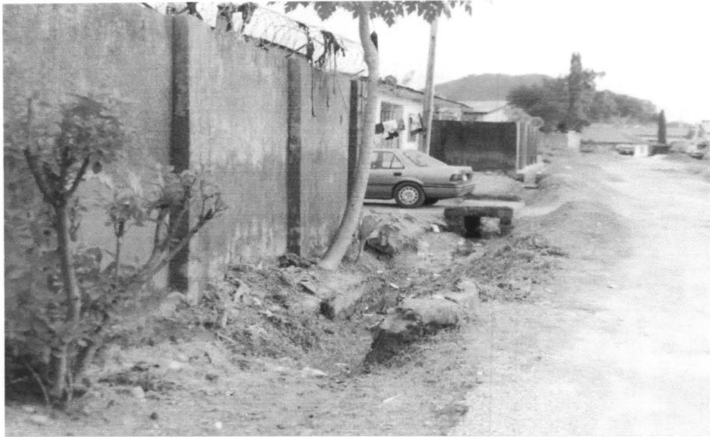
Plate I: Broken drainage gutter caused by constant flood in F.H.A. estate phase III Kubwa
