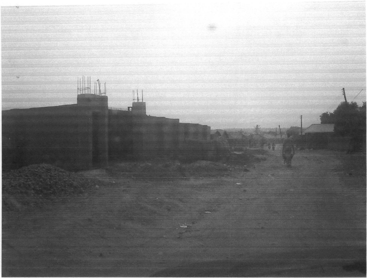
Plate IV: An on going blockwork building at Angwan waje; An area classified as Medium density
