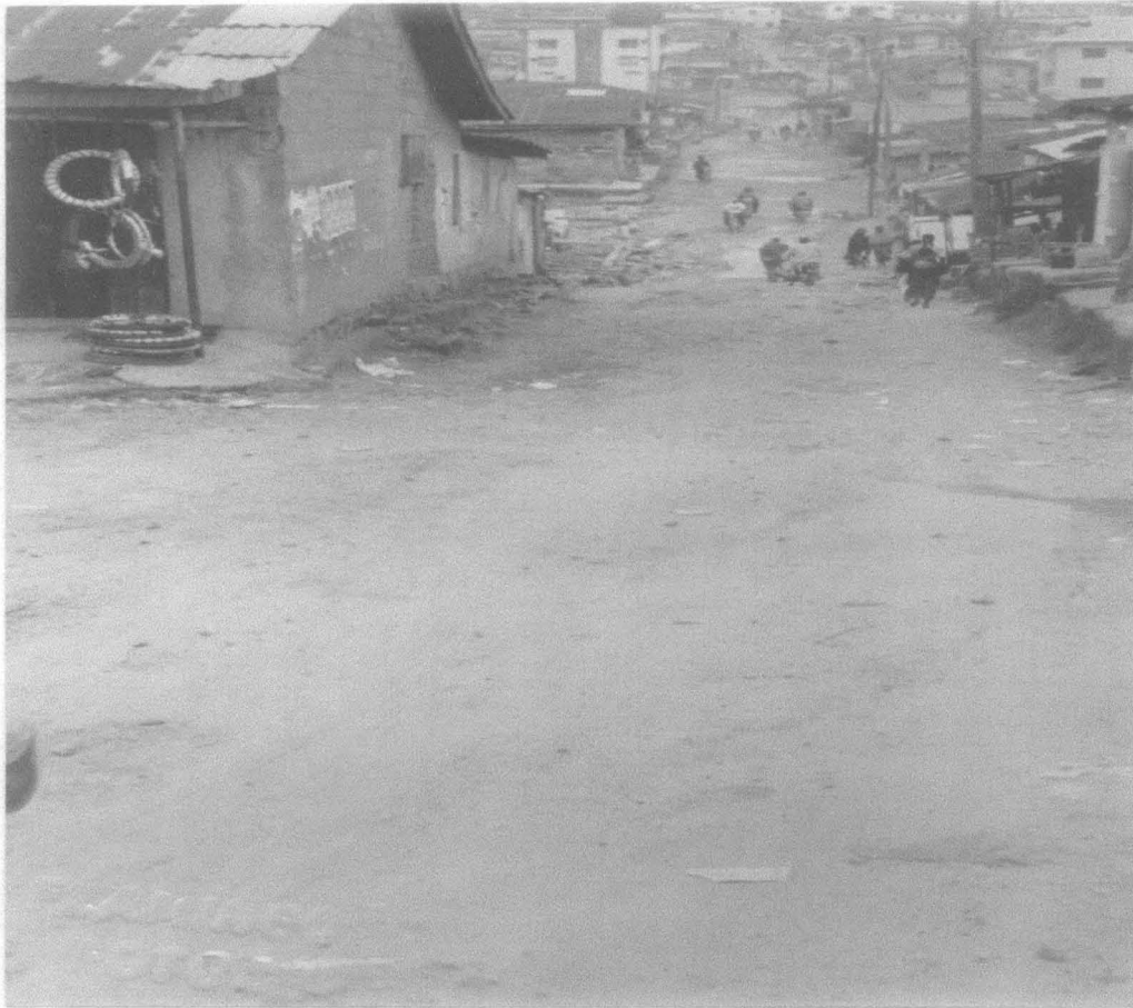
Plate 4.1b: Part of Victory Road in deplorable condition
