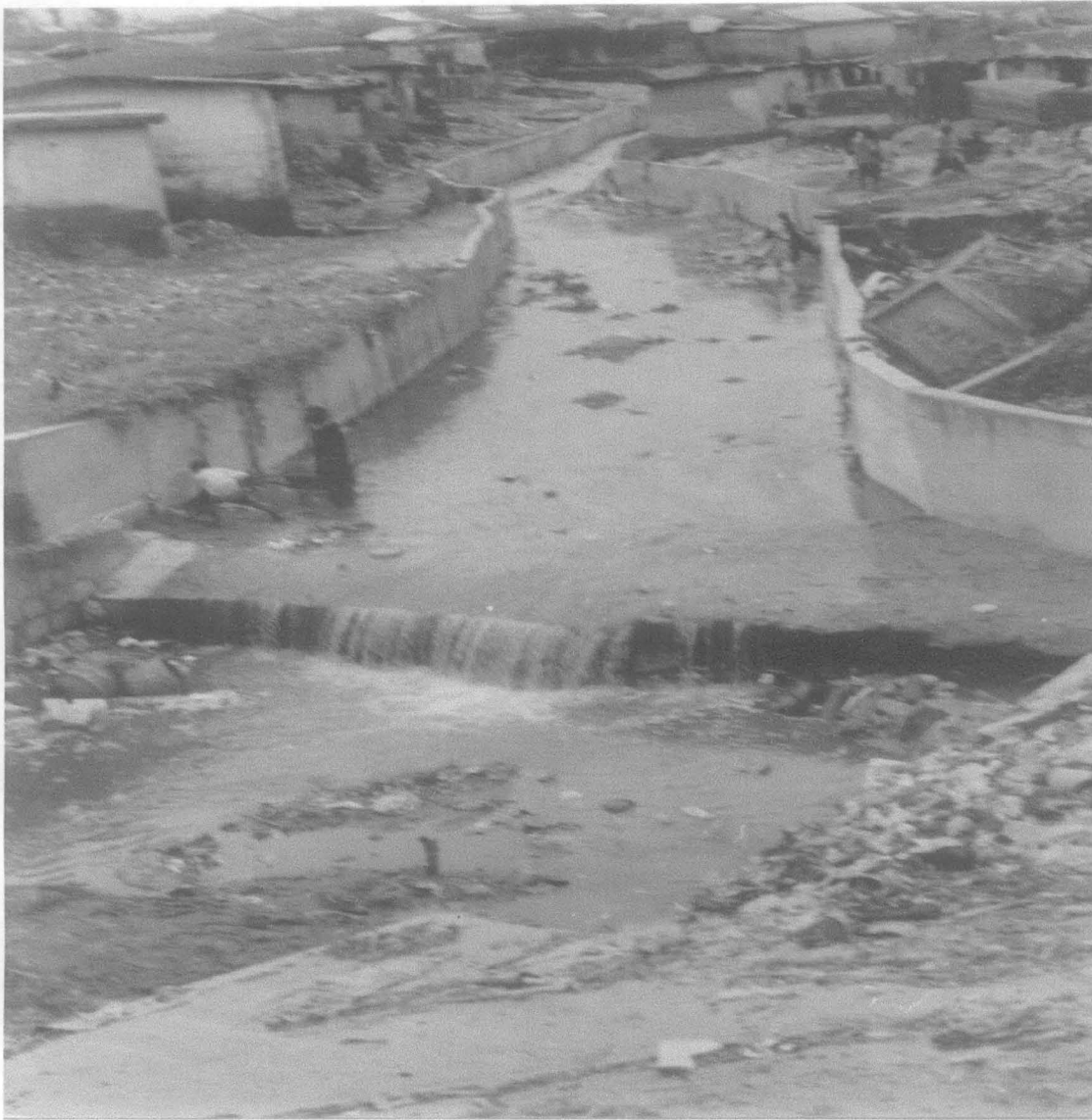
Plate 4.1f: Dawak Junction / U.B.A Road Water Channel, Drainage Banks not fully sandfill creating another vacuum for water pool.
