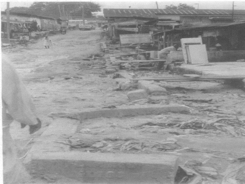
Plate 4.1c: Another Part of Victory Road completely devastated by erosion no longer motorable and road culvert blocked by deposits from unconstructed rainwater run off.
