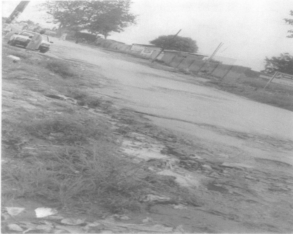
Plate 4.1d: GRA / Union Bank Road, washed away by Erosion, water storm channel not in existence
