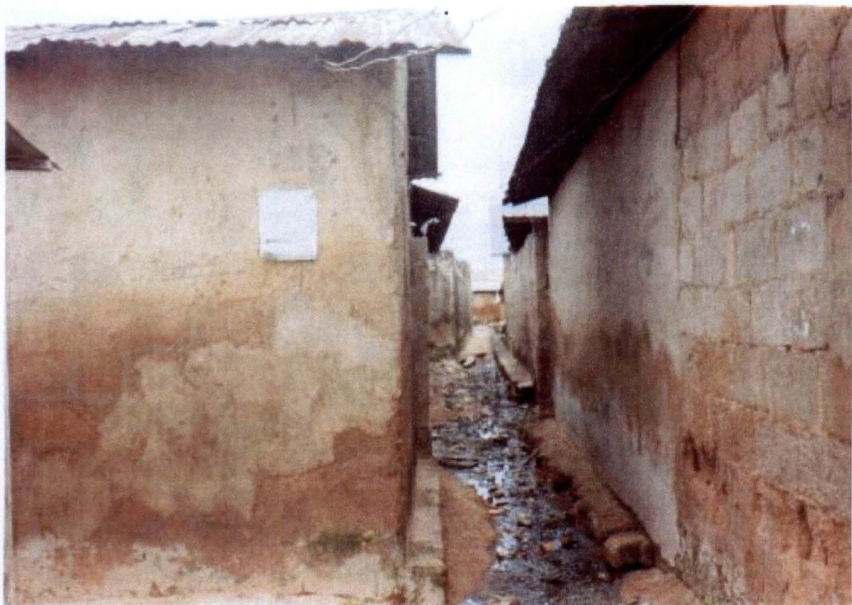
Plate IV: Showing inadequate drainage and poor spacing between buildings
