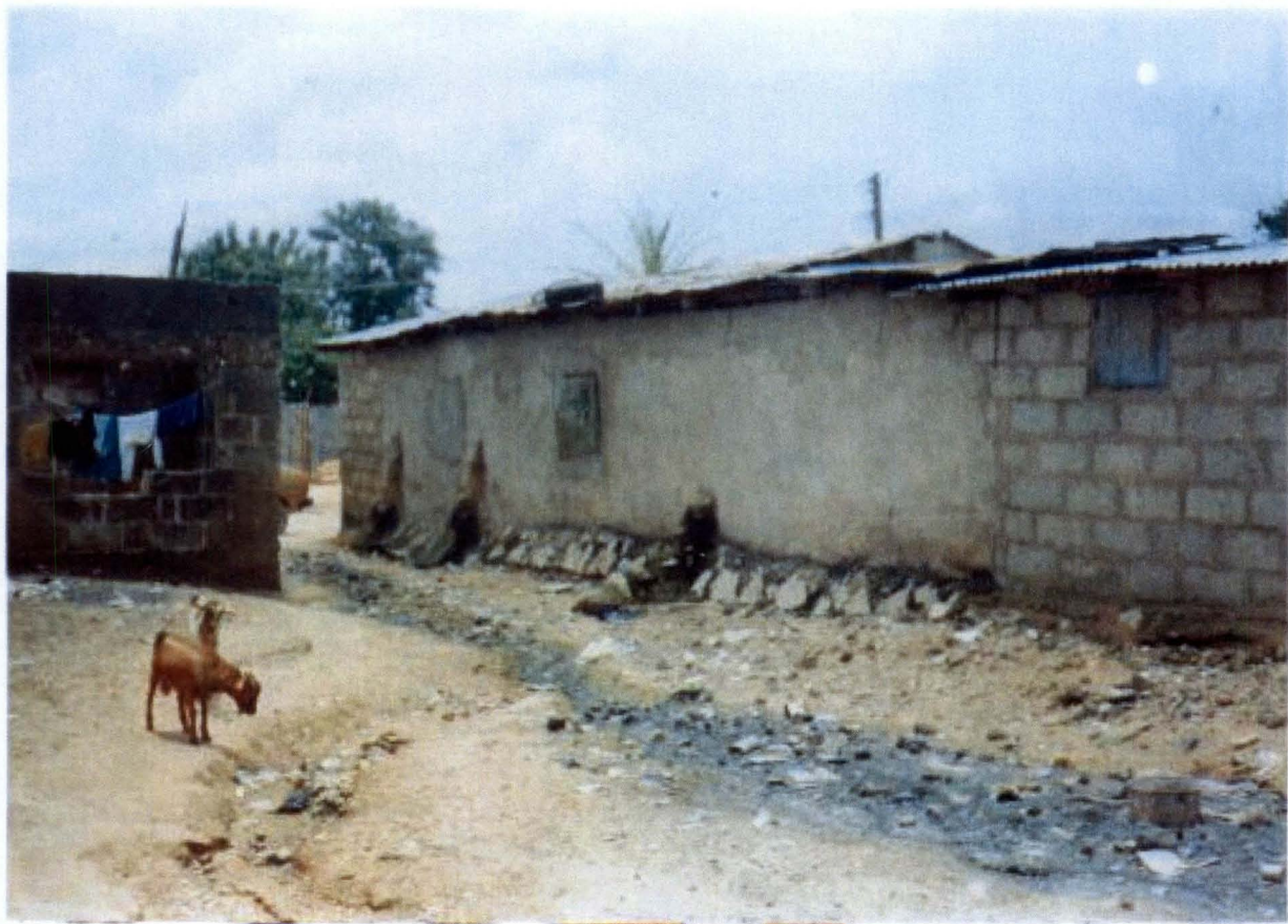
Plate VII: Showing a collapsed (but re-built) building
