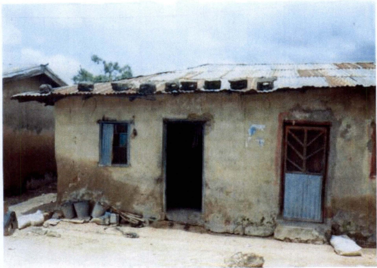
Plate III: Showing building whose roof is being threatened by wind/rainstorm
