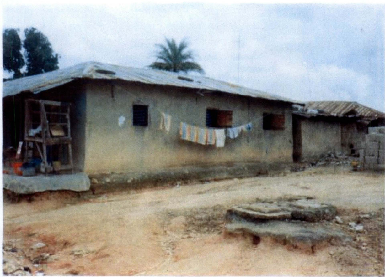
Plate I: Showing inadequate ventilation in a building studied
