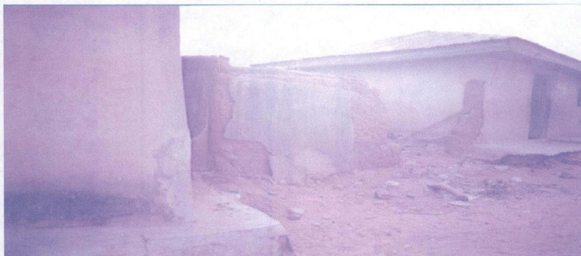
PLATE II DAMAGE BUILDING & FENCE - EMIN-NDASHABA
