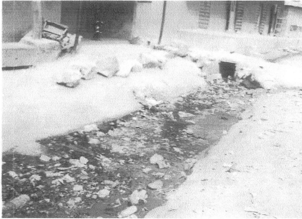
Plate I: showing drainage system in a residential
