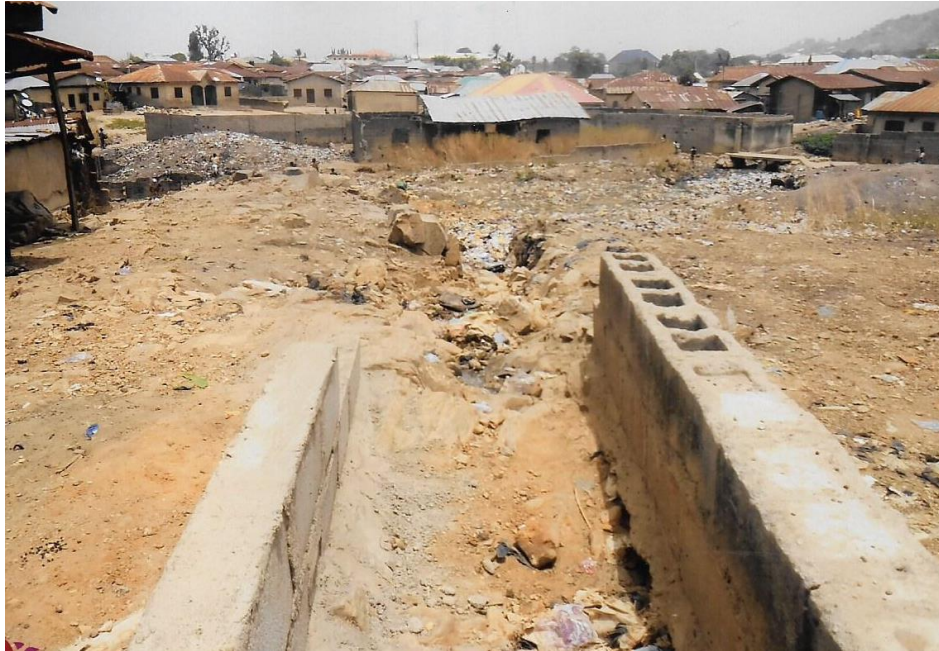
Plate IV: The condition of drainage in the area
