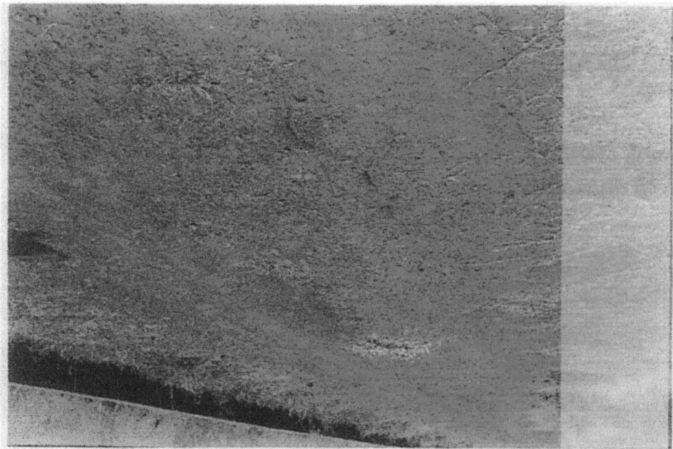
PLATE B:- Dam Embarkment with longitudinal crack at chainage 2.5km.
