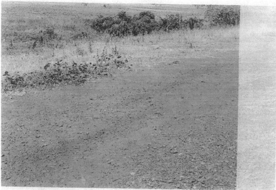
PLATE A:- Dam Embarkment with longitudinal crack at chainage 1.6km.
