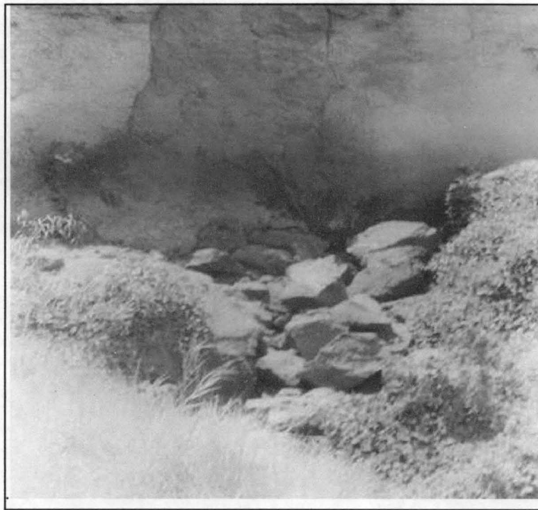
Plate 4.2: Expansion of sidewall
