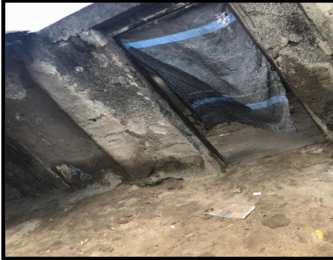
Plate IV: A cracked wall in the study area
