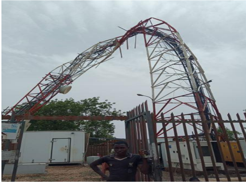
Plate IV: Sokoto tower collapse (Source: On site picture)
