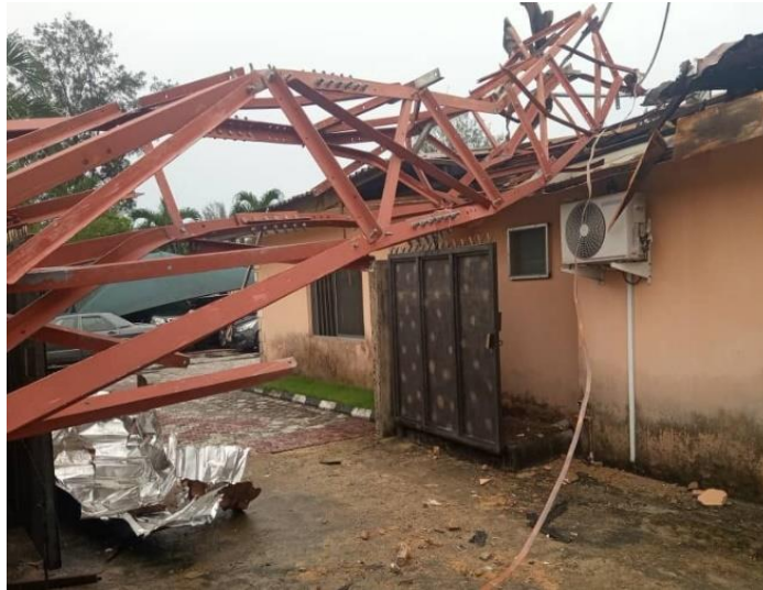
Plate VI: Akwa Ibom tower collapse II (Source: Abia, 2021)
