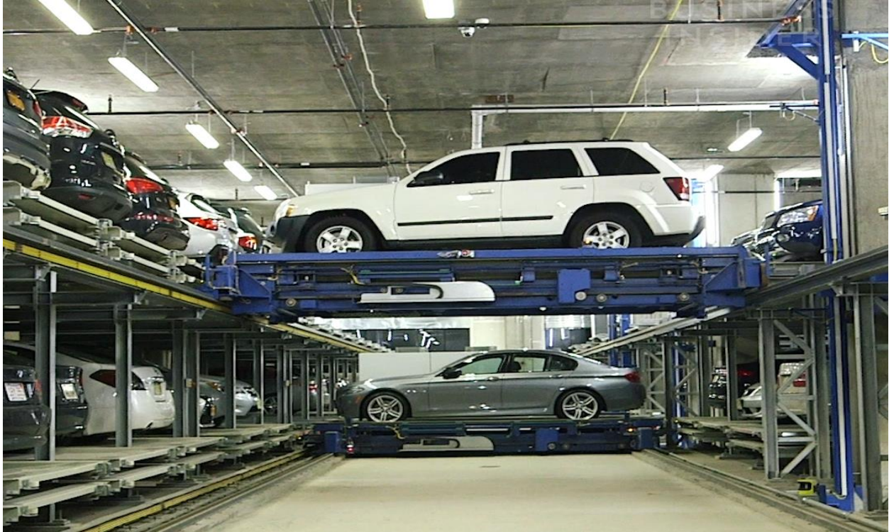
Plate 2.11: Automate Parking system in Liverpool
