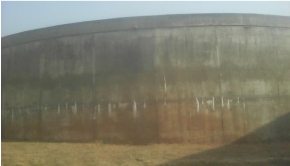
Plate IV: A clear water storage surface reservoir (Municipal Water Works, Minna)
