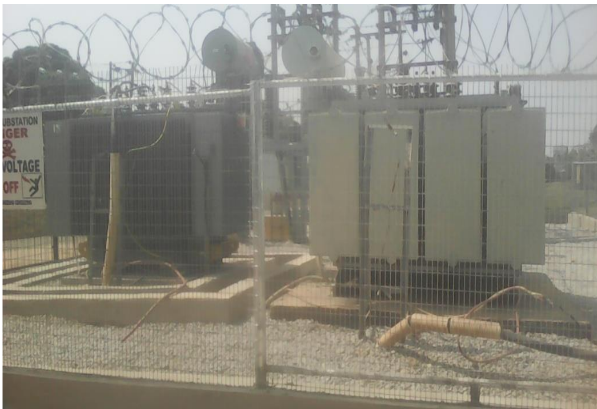
Plate VI: A step down Transformer deck (Municipal Water Works, Minna)
