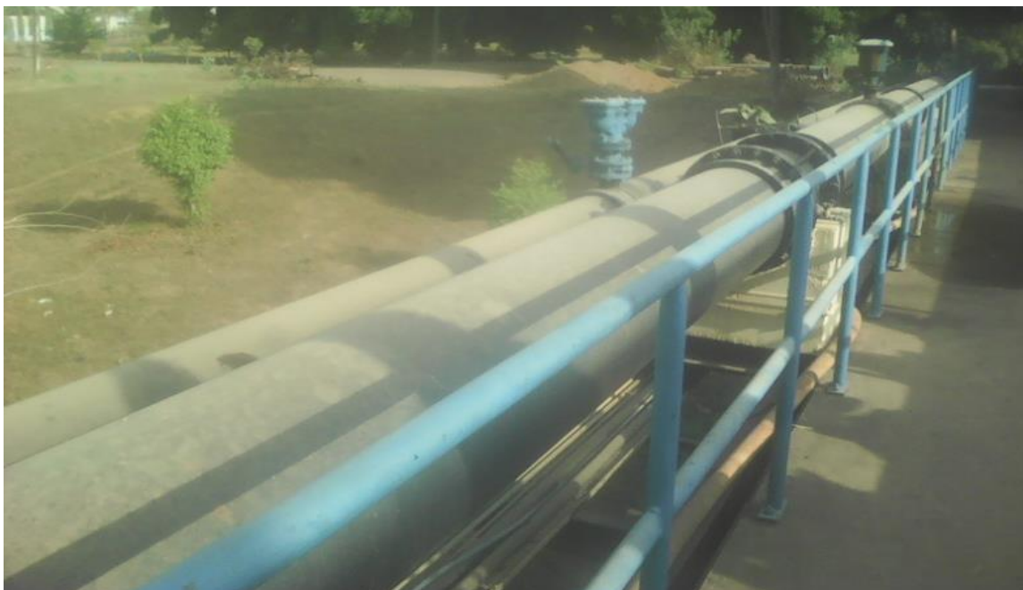
Plate II:: A Transmission system piping (Municipal Water Works, Minna)
