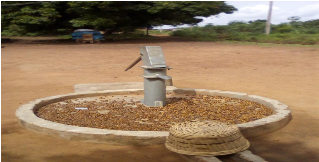
Plate 3: One of the non-functioning government sunk borehole at Alabi village
