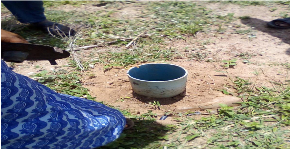
Plate 7: Uncompleted borehole water project by FADAMA in Gaa-sidi, Olorunsogo LGA
